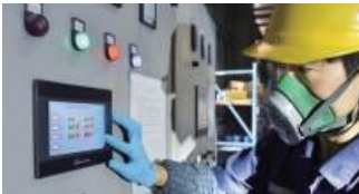
Waste gas environmental treatment 废气环保处理
